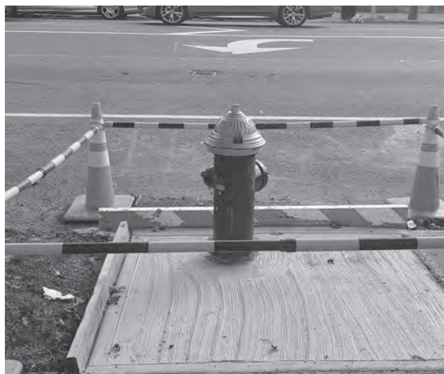
Second new fire hydrant standing tall.
