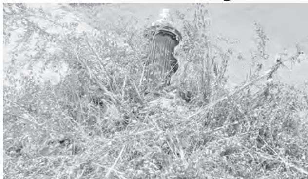
"Before" picture of fire hydrant covered in weeds and broken for three years
