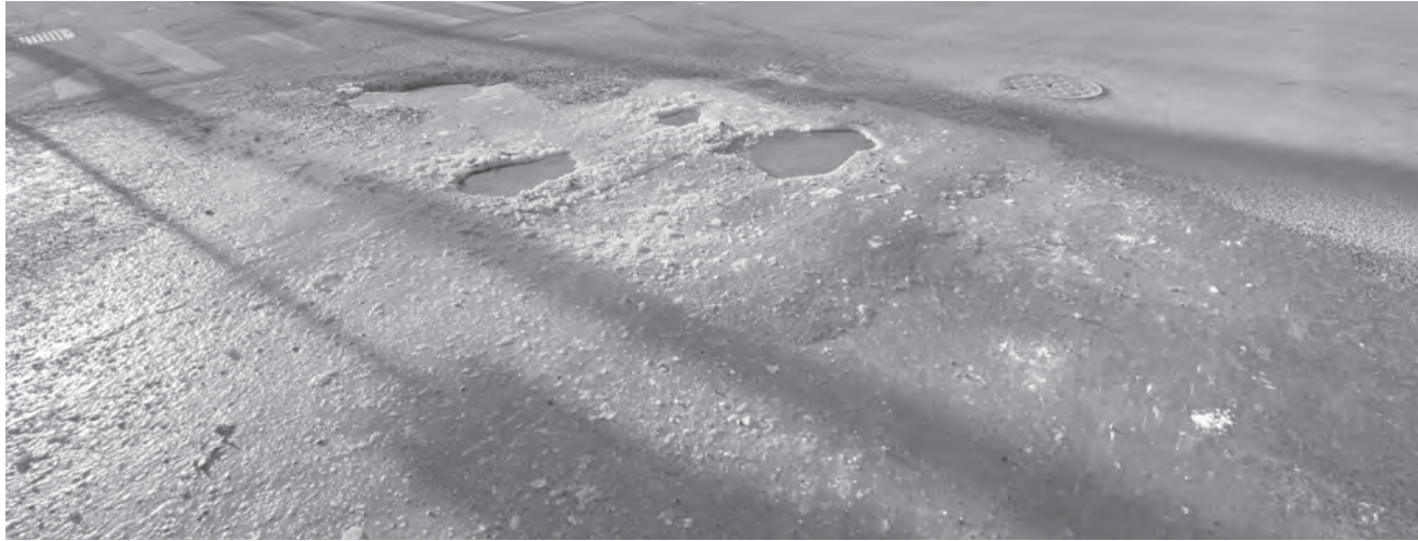
Large holes form at the intersection of Avenue K and East 105th Street.
