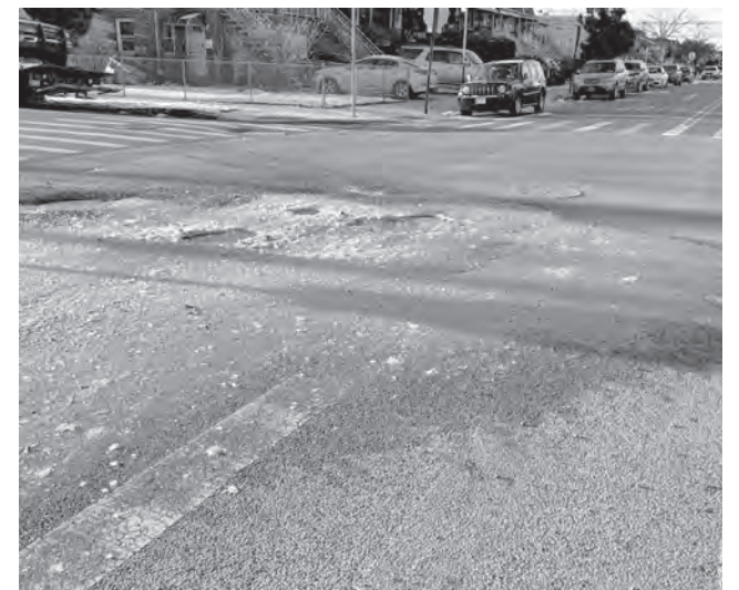
With freezing temperatures, the water turns to ice and slush.
